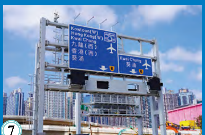
7 啟德交匯處連接路建造工程 Construction of connection roads of Kai Tak Interchange
