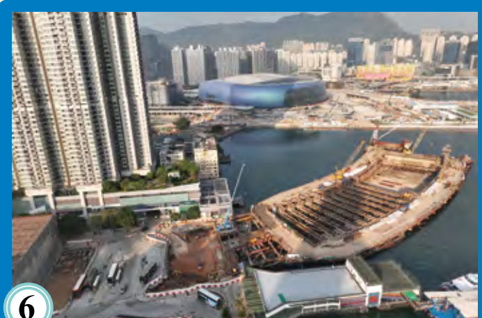
6 近馬頭角的第二期海底隧道回填工程 Backfilling works for stage 2 underwater tunnel near Ma Tau Kok
