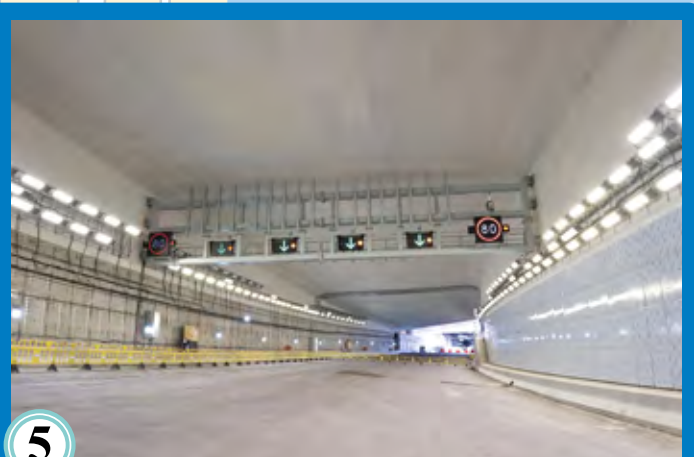
5 隧道機電、交通管制及監察系統安裝工程 Installation of electrical and mechanical, and traffic control and surveillance systems in tunnel
