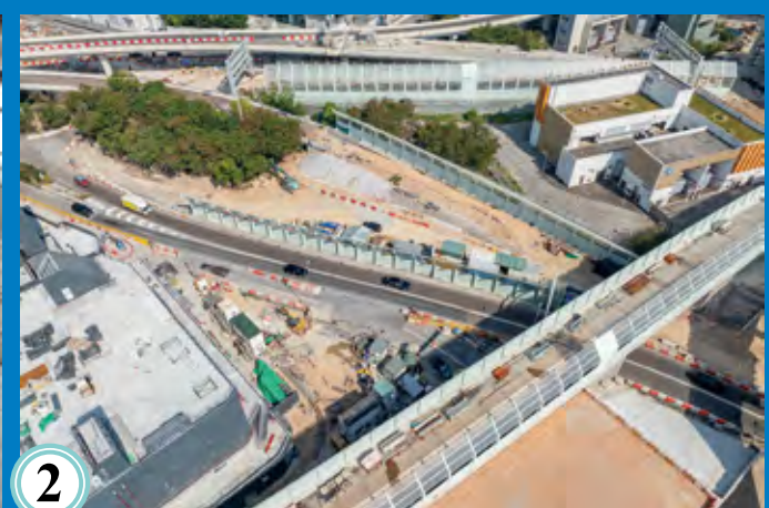
2 油麻地交匯處的隔音屏障建造工程 Construction of noise barriers at Yau Ma Tei Interchange
