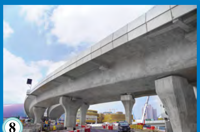
8 啟德交匯處行車橋護欄安裝工序 Installation of viaduct parapet wall at Kai Tak Interchange
