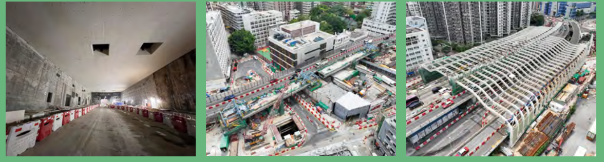
建造甘肅街明挖回填隧道 Construction of cut-and-cover tunnel at Kansu Street 重置加士居道天橋 Reprovisioning of Gascoigne Road Flyover 安裝加士居道天橋隔音罩 Installation of noise enclosure at Gascoigne Road Flyover
