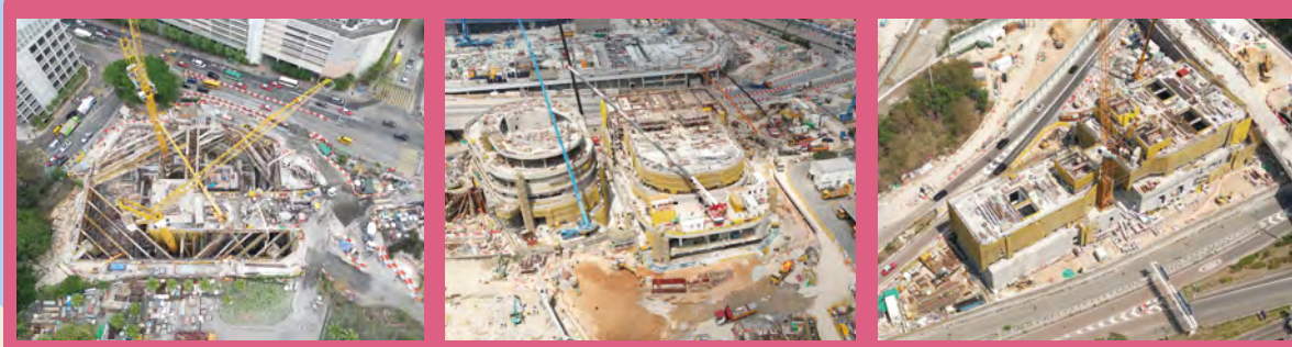
建造何文田通風大樓結構 Structural works of Ho Man Tin Ventilation Building 安裝啟德通風大樓及行政大樓的機電設備 Electrical and mechanical works and external works of Kai Tak Ventilation Building and Administration Building 安裝油麻地交匯處油麻地通風大樓的機電設備 Electrical and mechanical works and external works of Yau Ma Tei Ventilation Building at Yau Ma Tei Interchange
