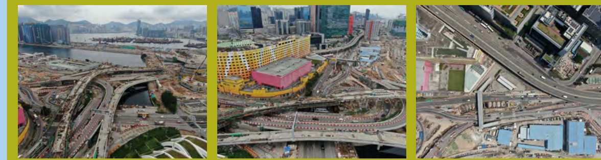
建造橫跨啟德河的行車天橋 Construction of vehicular bridges across Kai Tak River 建造橫跨啟福道的行車天橋 Construction of vehicular bridges across Kai Fuk Road 建造啟福道的地下行車道 Construction of underpass at Kai Fuk Road
