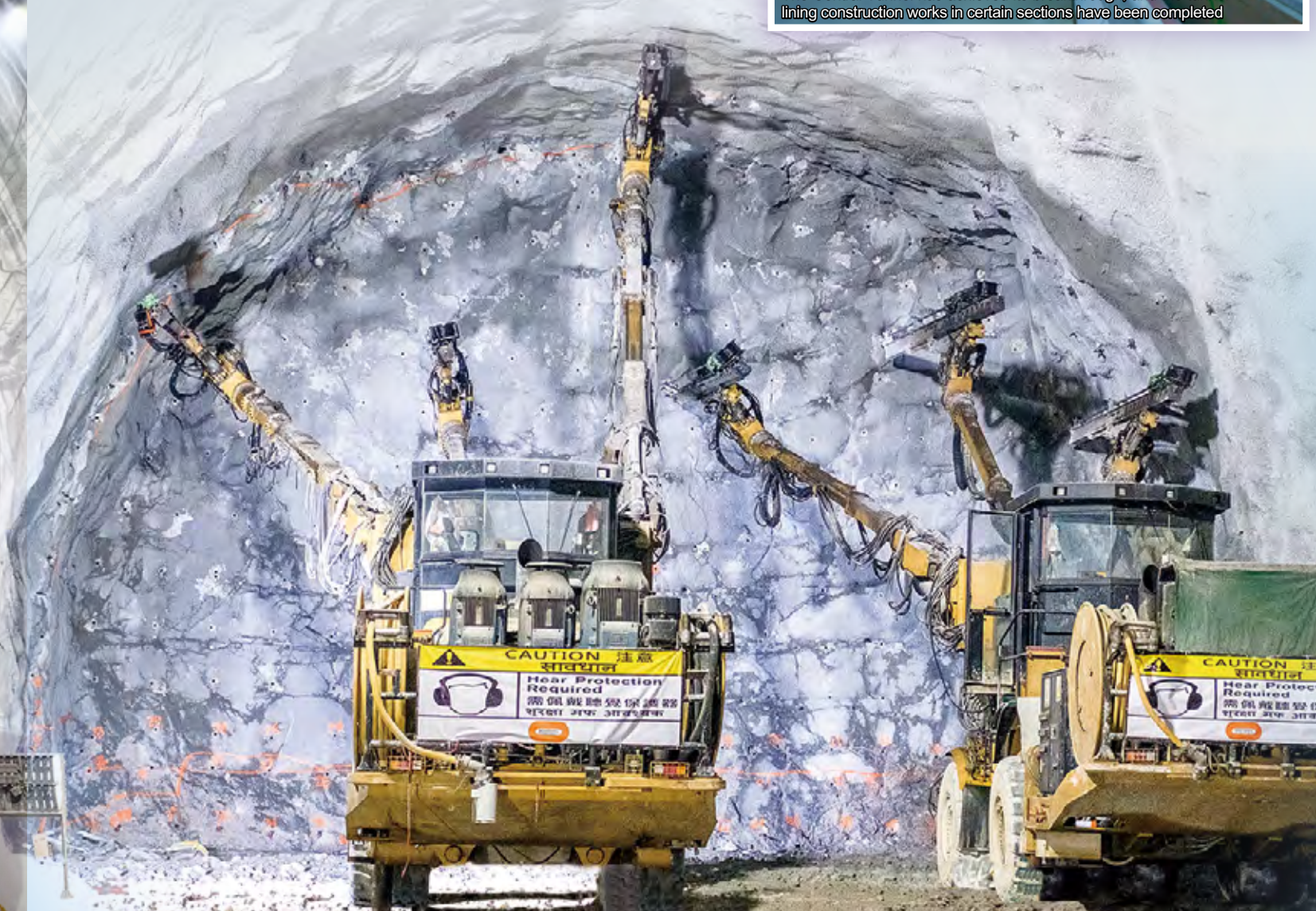
中段隧道鑽孔工程的炮眼孔序 Blast hole drilling process of the Central Tunnel drill-and-blast works. Photographer: Mach Lai@2021 All Right Reserved
