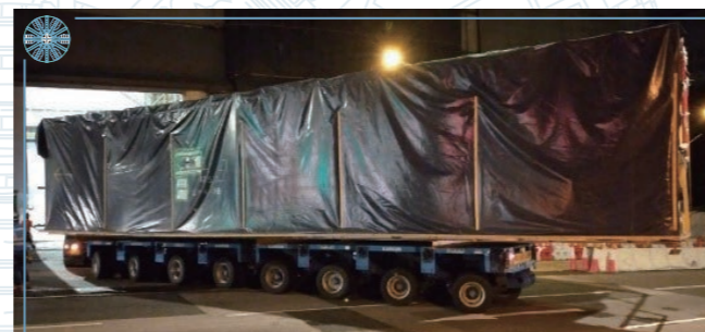
隧道鑽挖機組件由陸路運送到何文田工地 Components of TBM finally delivered to Ho Man Tin site by land
