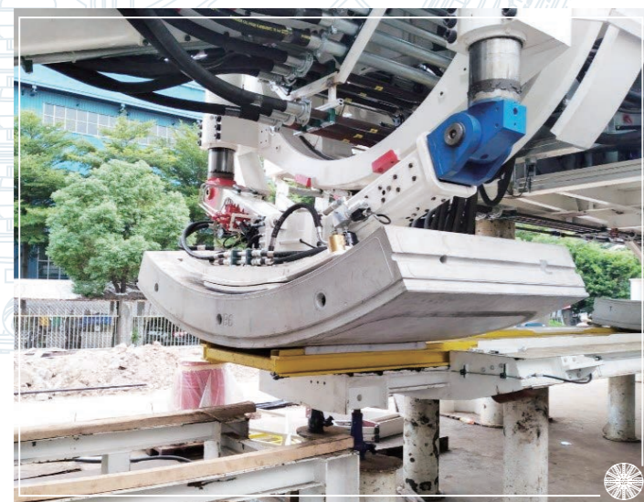
隧道鑽挖機在鑽挖的同時安裝隧道襯砌預製組件 TBM installs precast tunnel lining segments at the same time as it bores
