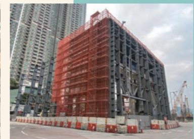
於馬頭角豎井通道工地興建臨時隔音罩 Construction of temporary noise enclosure is in progress at Ma Tau Kok access shaft works site
