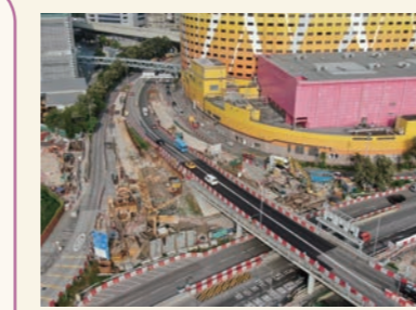
橫跨啟祥道的行車天橋鑽孔樁工程 Bored piling works for vehicular bridges across Kai Cheung Road
