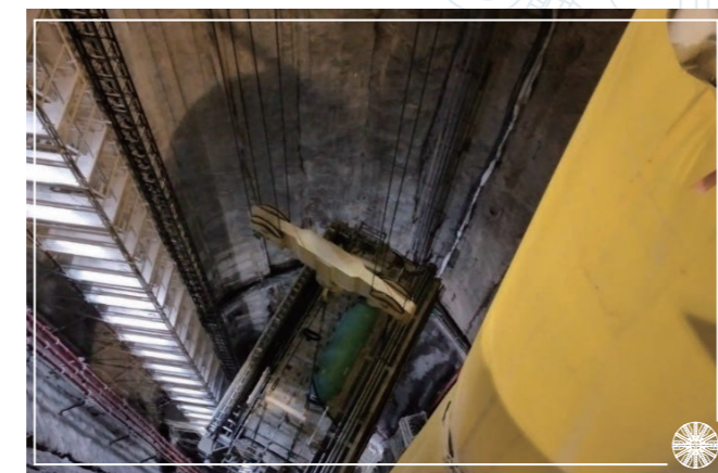
隧道鑽挖機組件吊到豎井通道下進行組裝 Components of TBM were lifted down to the tunnel via access shaft and assembled in the tunnel
