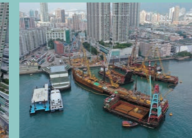
在九龍灣的第二期海底隧道的臨時海上工作平台及圍堰建造工程 Installation of temporary marine platform and construction of cofferdam for Underwater Tunnel Stage 2 at Kowloon Bay
