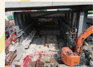
於油麻地豎井通道工地興建臨時隔音罩 Construction of temporary noise enclosure is in progress at Yau Ma Tei access shaft works site
