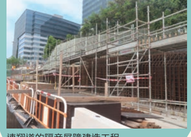
連翔道的隔音屏障建造工程 Noise barriers construction at Lin Cheung Road
