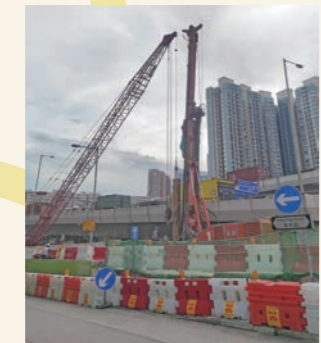
渡船街天橋隔音屏障建造工程 Noise barriers construction on Ferry Street Flyover
