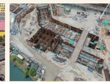
地下行車道、通風及機電坑道的結構建造工程 Construction of underpasses, ventilation and electrical and mechanical adit
