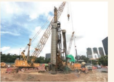
油麻地通風大樓的嵌岩鋼工字樁安裝工程 Pre-bored socketed H-pile installation works at Yau Ma Tei Ventilation Building works site
