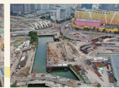
橫跨啟德河的行車天橋鑽孔樁工程 Bored piling works for vehicular bridges across Kai Tak River
