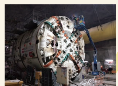
於何文田隧道內組裝隧道鑽掘機 Assembly of TBM inside tunnel
