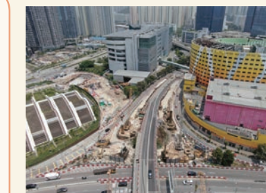
橫跨啟祥道行車天橋的鑽孔工程 Bored piling works for vehicular bridges across Kai Cheung Road
