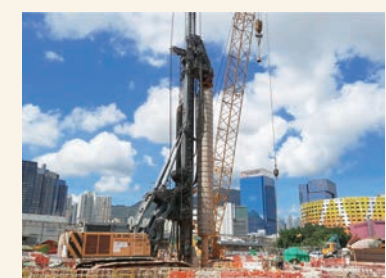
啟德通風大樓及行政大樓的嵌岩鋼字樁安裝工程 Socketed H-pile installation works at Kai Tak Ventilation Building and Administration Building works site
