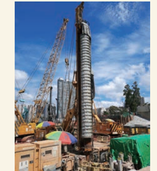
油麻地通風大樓的嵌岩鋼字樁安裝工程 Socketed H-pile installation works at Yau Ma Tei Ventilation Building works site
