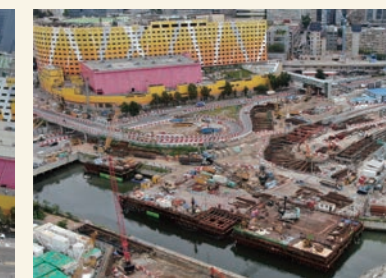
橫跨啟德河行車天橋的鑽孔工程 Bored piling works for vehicular bridges across Kai Tak River
